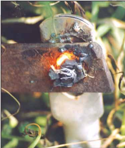
Improper lug connection resulting in heating up
