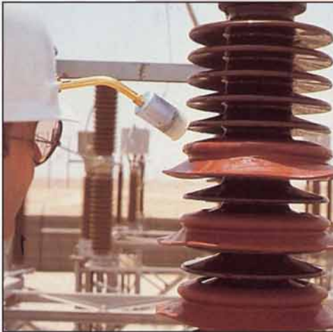
Raychem's Creepage extender installed on a insulator
