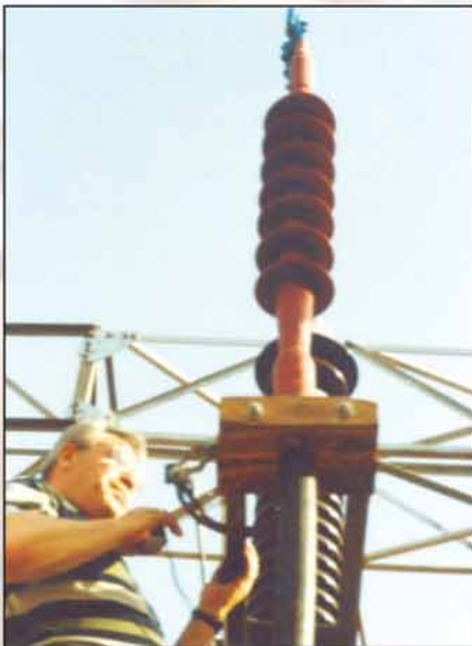
66kV XLPE Outdoor Termination installed in Gujarat Electricity Board, Vadodara
